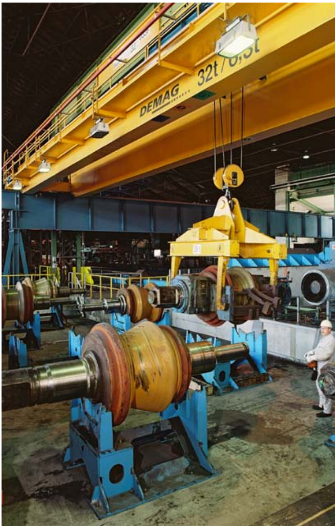
32/6.3-t two-girder overhead travelling crane for roll-changing in a plant making sheet piling
