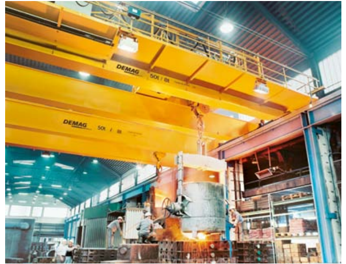
Two 50/8-t two-girder overhead travelling cranes for transport of ladles and flasks in Germany, span 17 m
