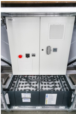
41583-13: Demag control with batteries
